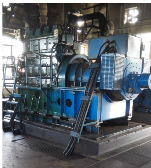
Figure 6: Old diesel generator at Ngara
